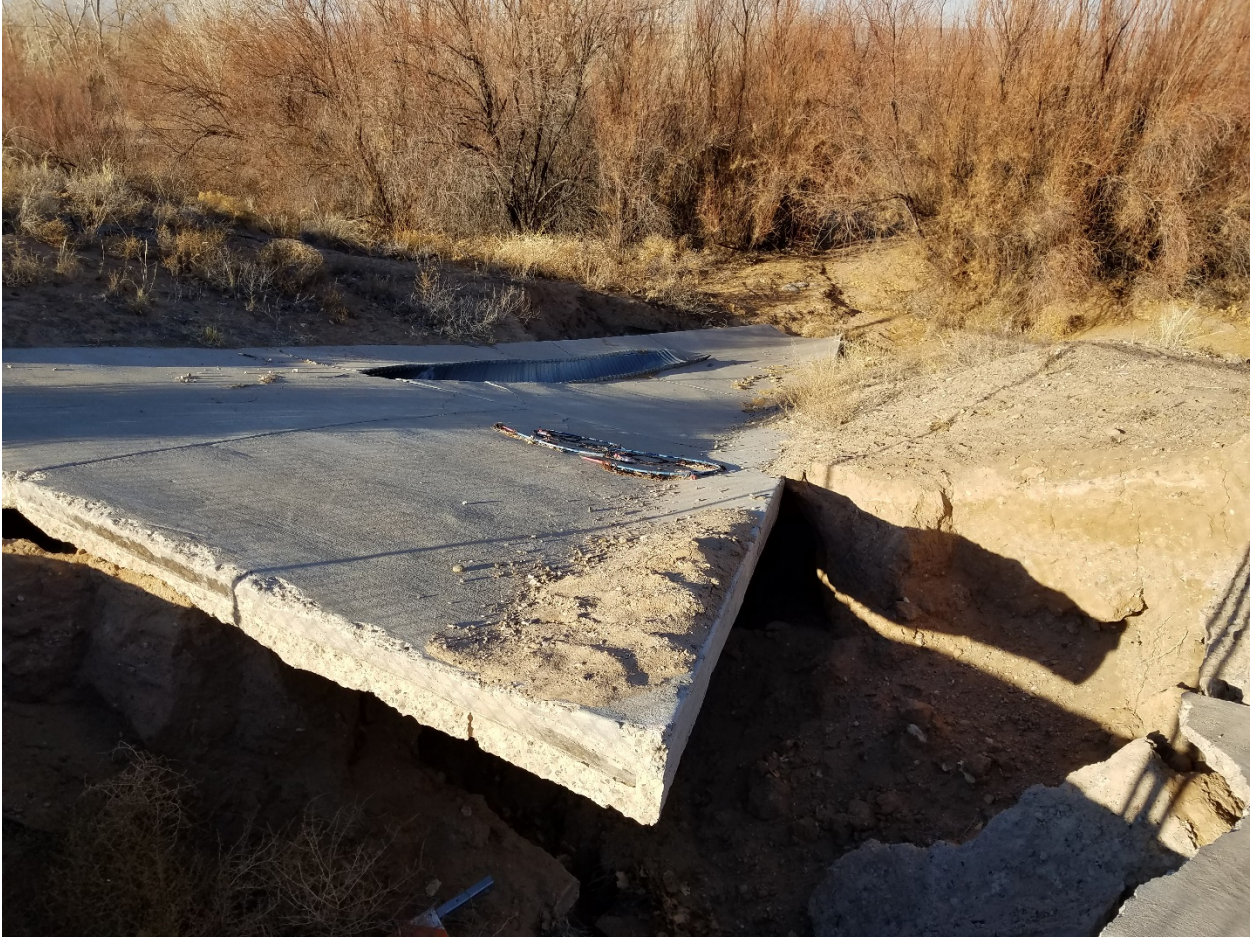
Concrete rundown: Detail of damaged
