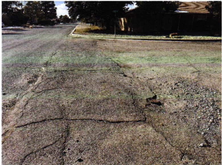
Figure 4: Fatigue (Alligator) cracking
