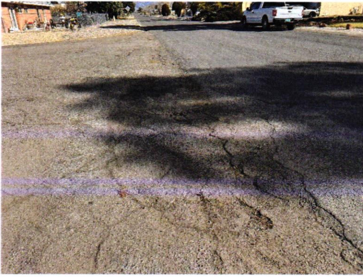
Figure 3: Fatigue (Alligator) cracking
